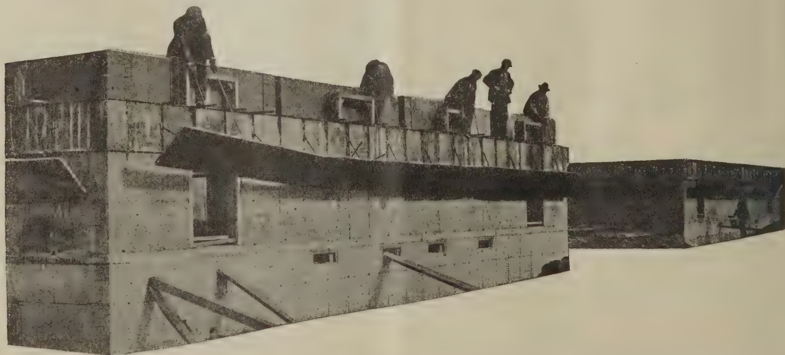
A CONCRETE WALLED HOUSE IN COURSE OF CONSTRUCTION. RAISING THE METAL FORMS FOR POURING THE NEXT TIER OF CONCRETE WALL. THESE FORMS ARE HINGED AND SWING UP WITH COMPARATIVE EASE
